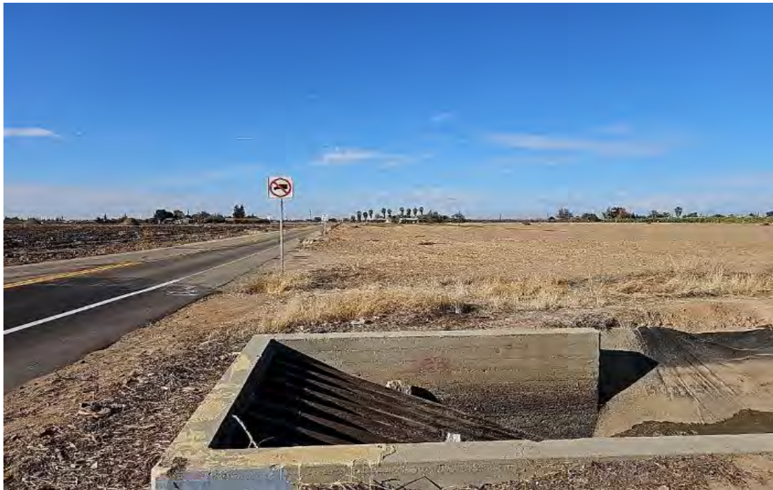
Figure 9. Photograph from the southeast corner of the Project site, looking west, showing Horsman Ditch as it enters a box culvert under West Sierra Way.
